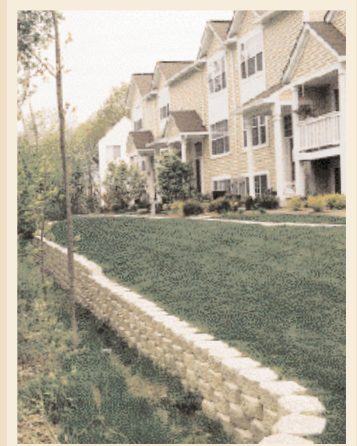
This short yet effective retaining wall was installed by Fisher Burton to support and confine the lawns of a townhome development bordering a wooded area.
