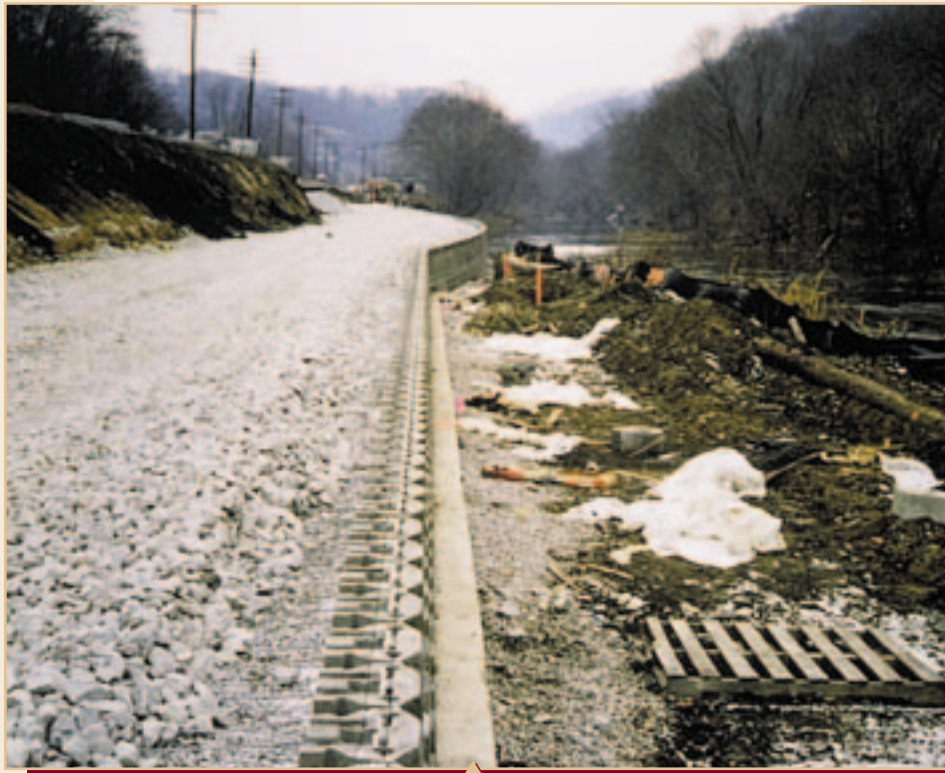
Wall Under Construction - Concrete Leveling Pad, Curved Geometry and Select Drainable Backfill
