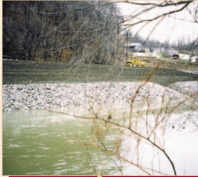
View of Flood Wall with Rip Rap at Toe to Prevent Base Scour
