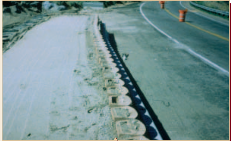
Falling rock barrier - Keystone wall facing the road, with reinforced soil zone behind, backed by wall of old tires.
