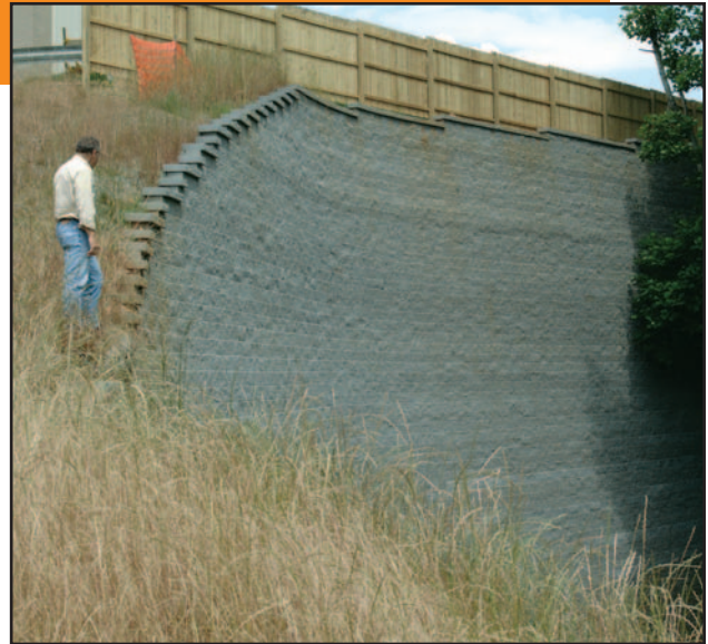
With the help of geosynthetic reinforcement, Square Foot Retaining Walls can be built more than 40 feet tall. — Gainesville, Ga.
